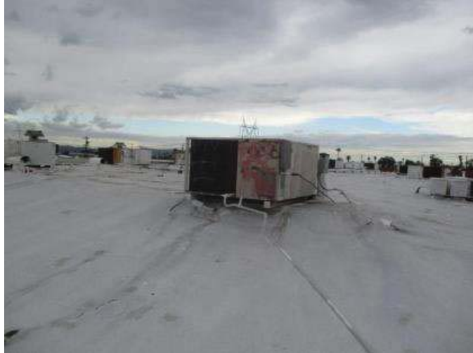
The heating and cooling units are located on the roof.
