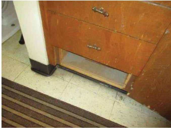
The bathroom cabinet is damaged.
