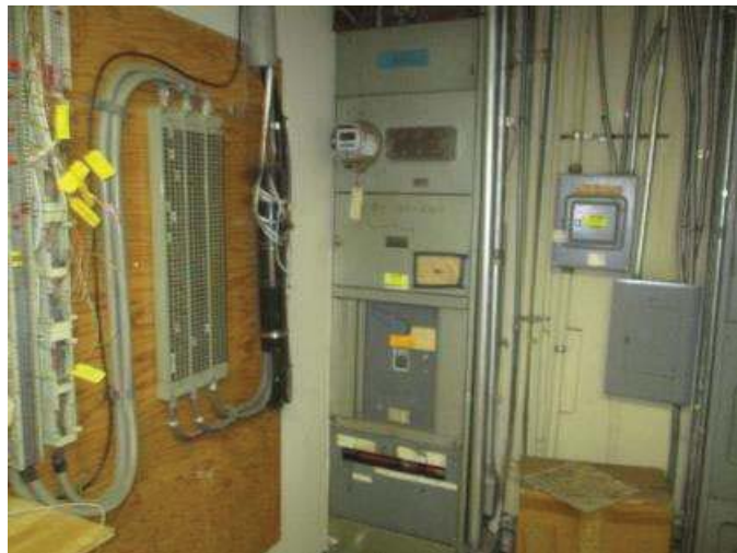
The main electrical supply panel is in an electrical room inside the building.
