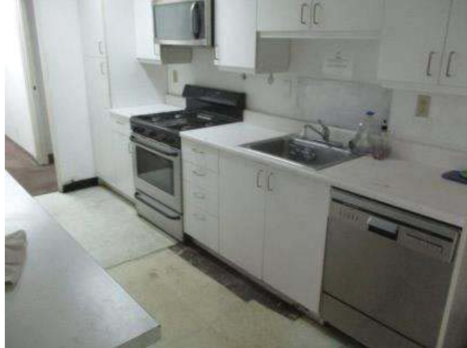
This kitchen is showing excessive wear.
