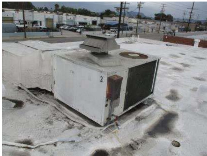
The heating and cooling systems for the building are known as "Roof Packages". This is the type of system where the gas heating furnace and the electric air conditioning (cooling) components are packaged inside one container and perform both functions from this common location on the roof.
