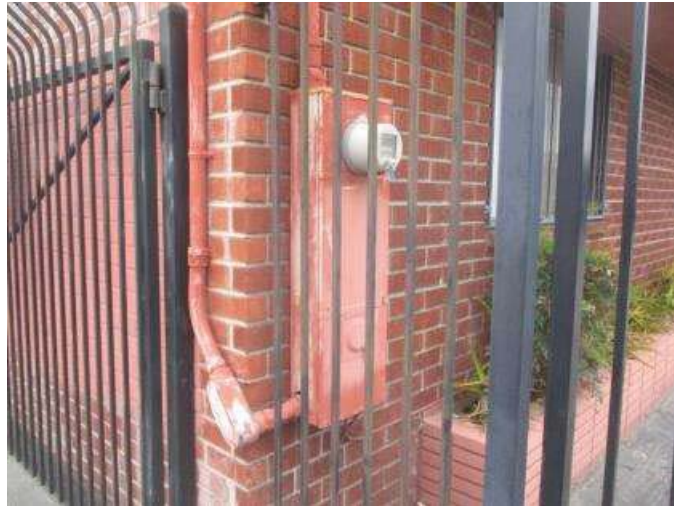
The main electrical panel is located on the front exterior of the building.
